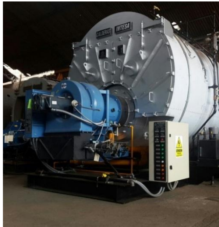
Figura 16: Caldera pirotubular 800 BHP
