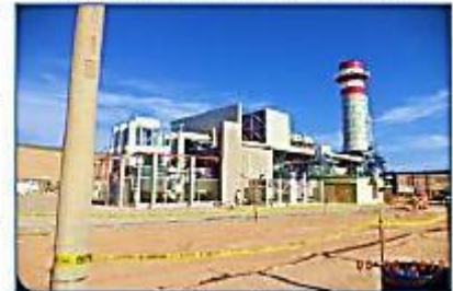
Turbina a gas (TG2)
