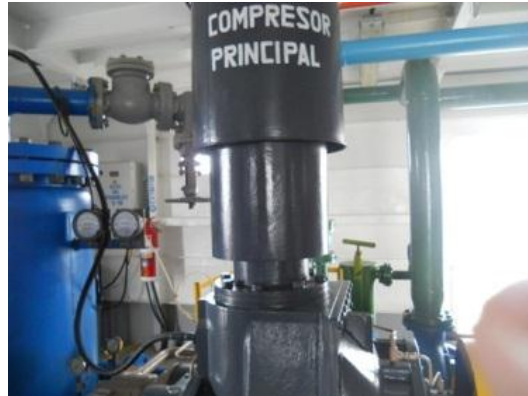
Figura 2.7: Compresor principal (tornillo)
